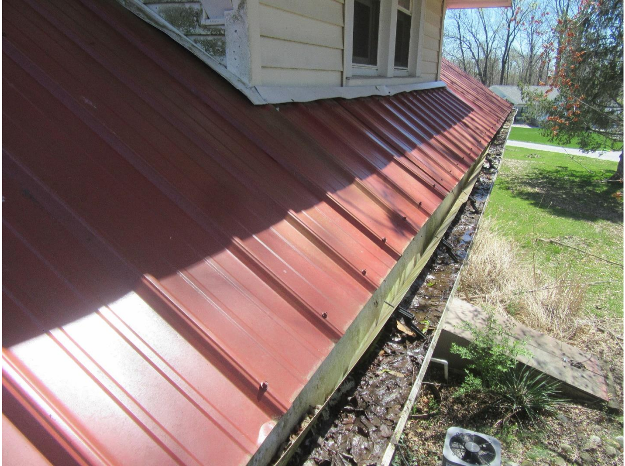
#19 View along the lower west side. The gutter is loose and pulling away from the house.
