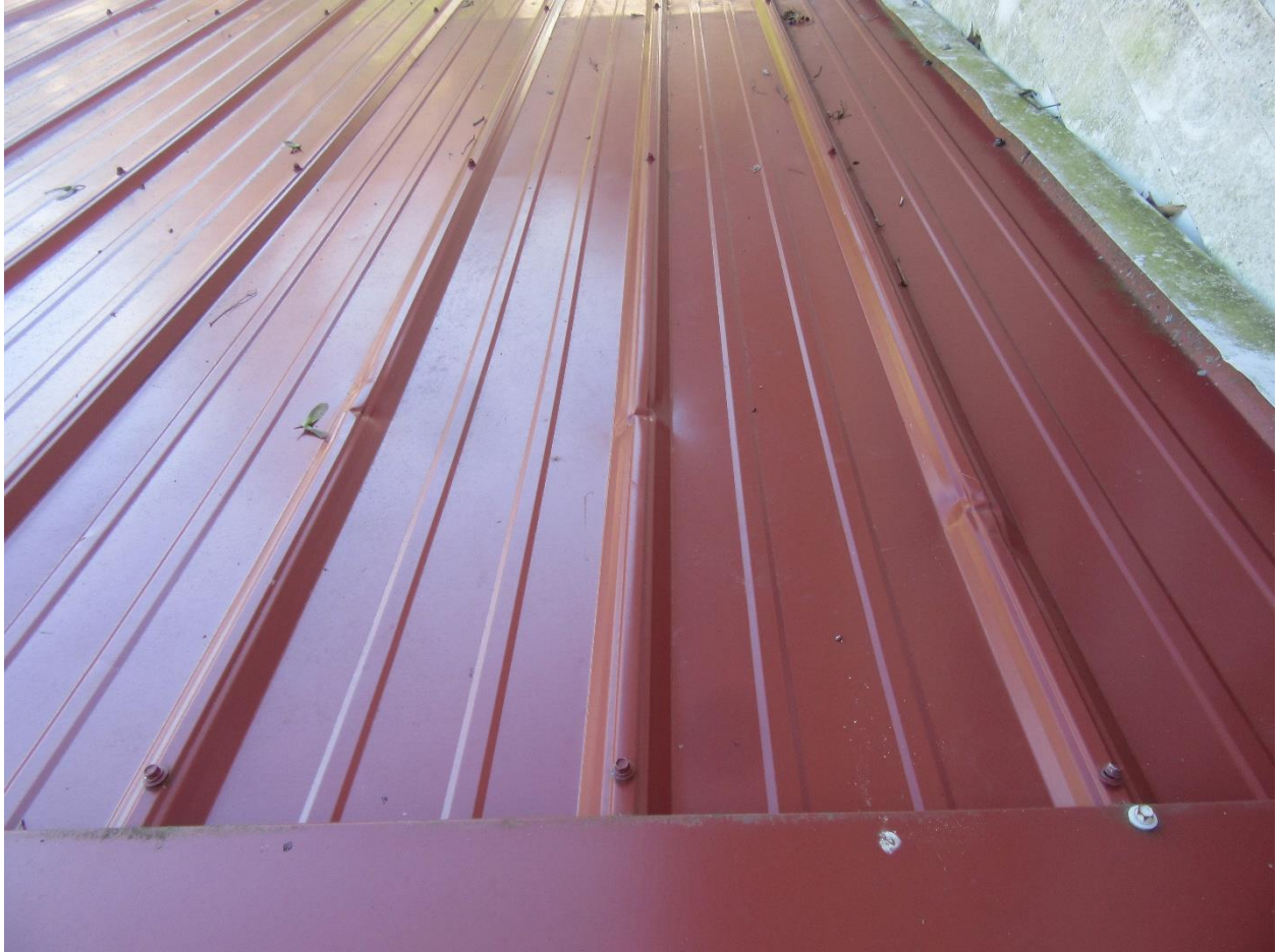
#7 Some of the dents on the front porch roof metal panels.
