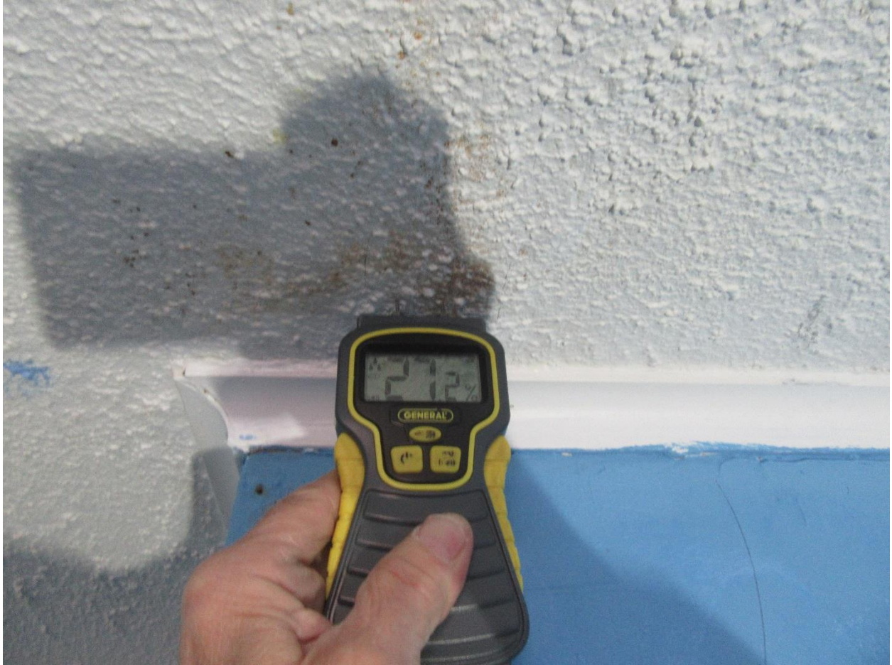
#33 Elevated moisture level reading on the upper level bathroom ceiling. The chimney is located behind the wall.
