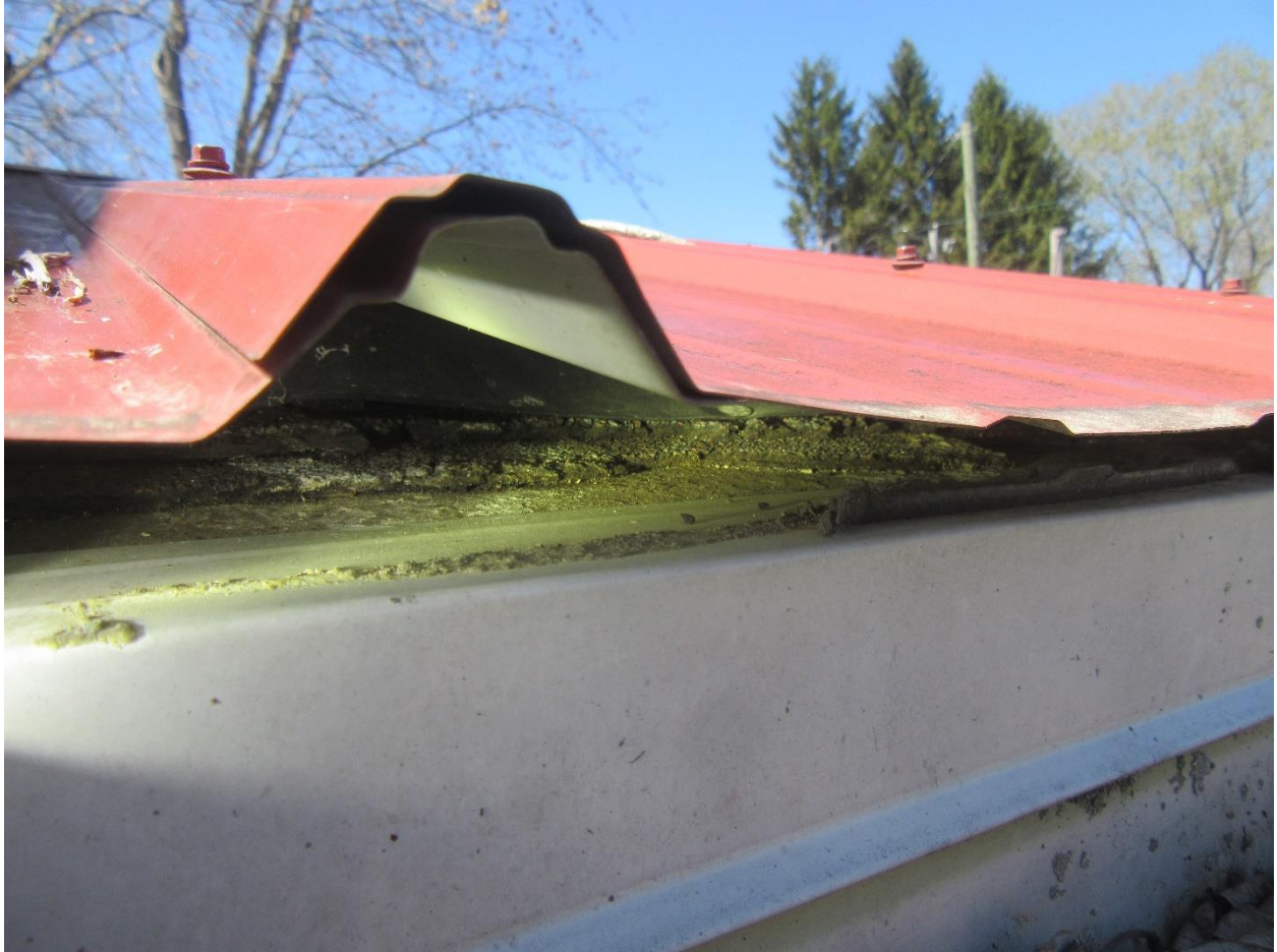
#15 View along part of the lower edge of the metal roof. (See next photo)
