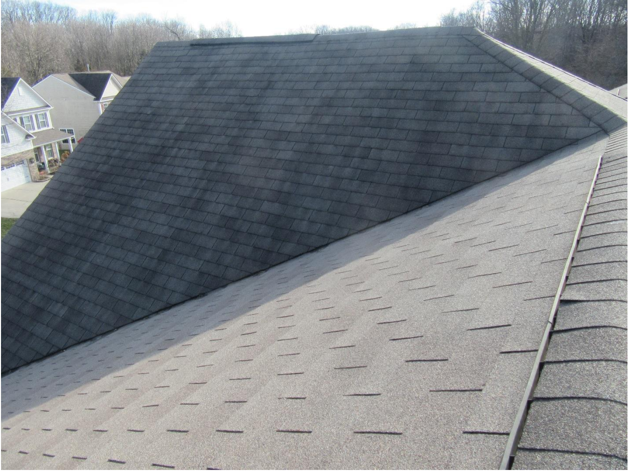
#9 View of the upper front center area. Some algae is growing on the steep roof area.
