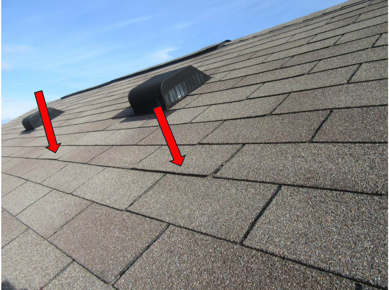
#16 A few shingle tabs on the back side are slightly raised and loose.
