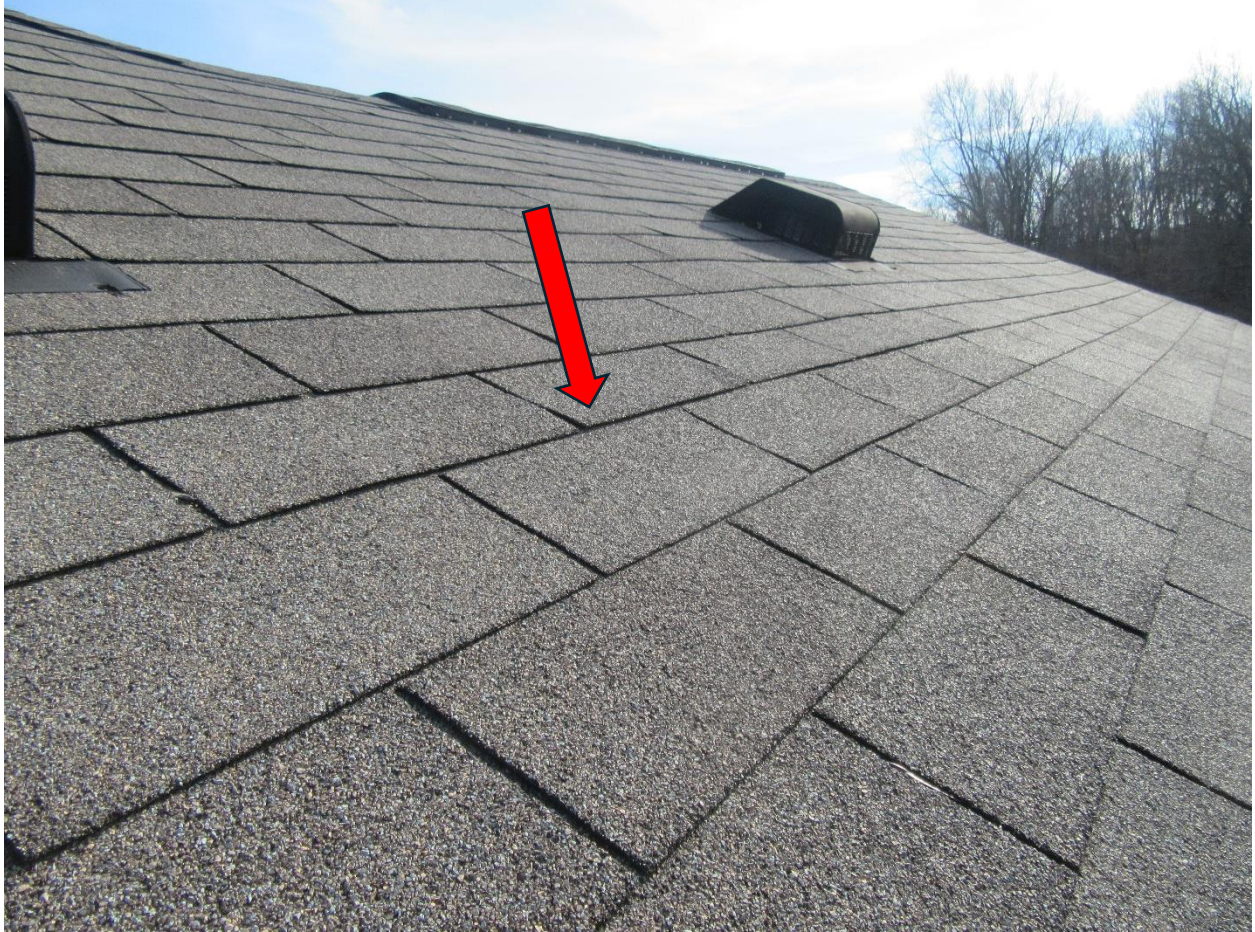
#18 A few shingle tabs on the back side are slightly raised. (See comments in previous photos)
