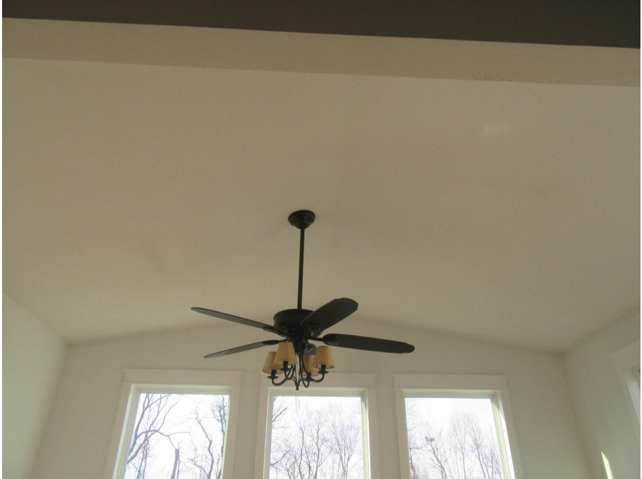
#28 View of the main level back room ceiling. The small lower back roof is directly above this room.
