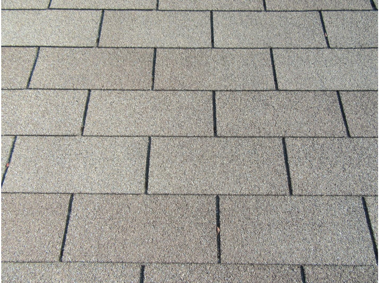
#15 Close-up view of some shingles. Shingles appear to be in satisfactory condition for their age.
