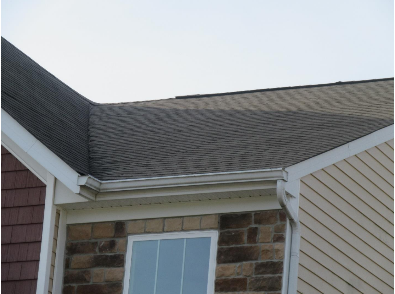
#23 View of the upper front N/E corner roof area. A few shingle tabs have slightly raised edges.
